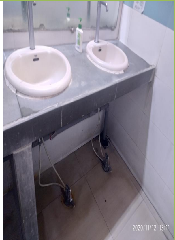
College can adopts hands free water taping system. This saves the water and also good for personal health protection to avoid frequent hand touching to water taps.
